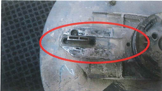
Highlighted in red where adjustments bolts came loose
