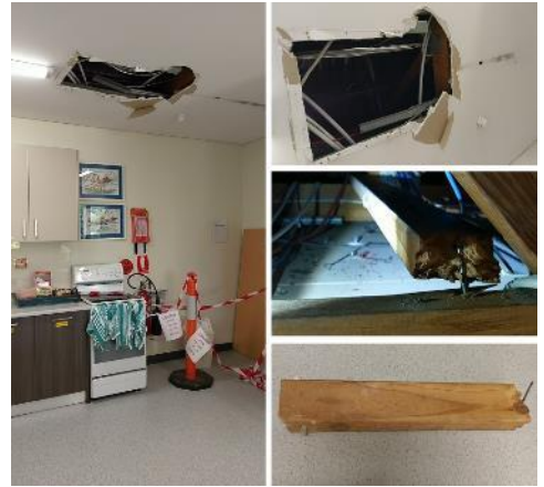
Gyprock Ceiling and Broken Timber
