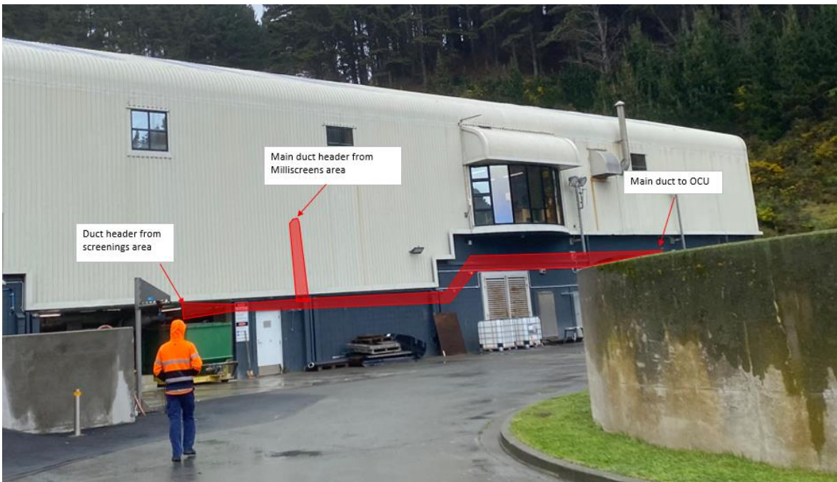
Figure 3-22: Option 2b (AC, BTF and BTF+AC) Main header to the north of building
