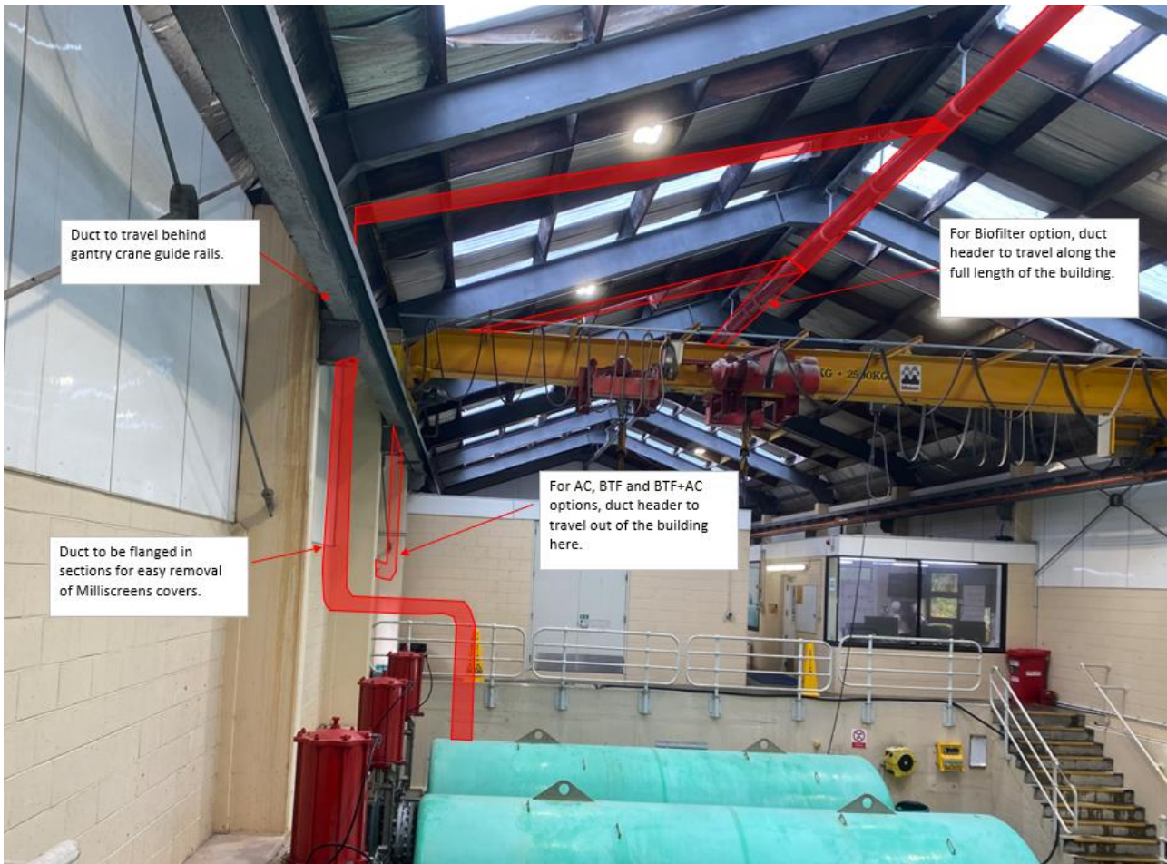
Figure 3-4: Milliscreens ductwork (only one shown) and main duct header.
