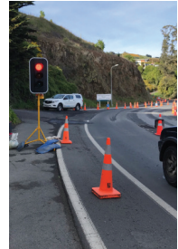
Operator can now stand safely away from the eSTOP. Use handset to change signals as required
