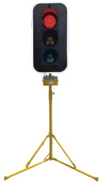
Use handset to test operation of each phase of the lantern. Set lantern to Go, then to Stop
