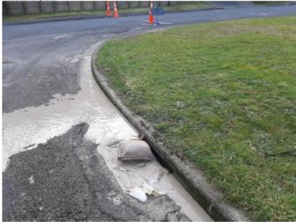
Figure 1: Sediment laden water entering the stormwater sump on Hair Street with inadequate sediment controls in place
