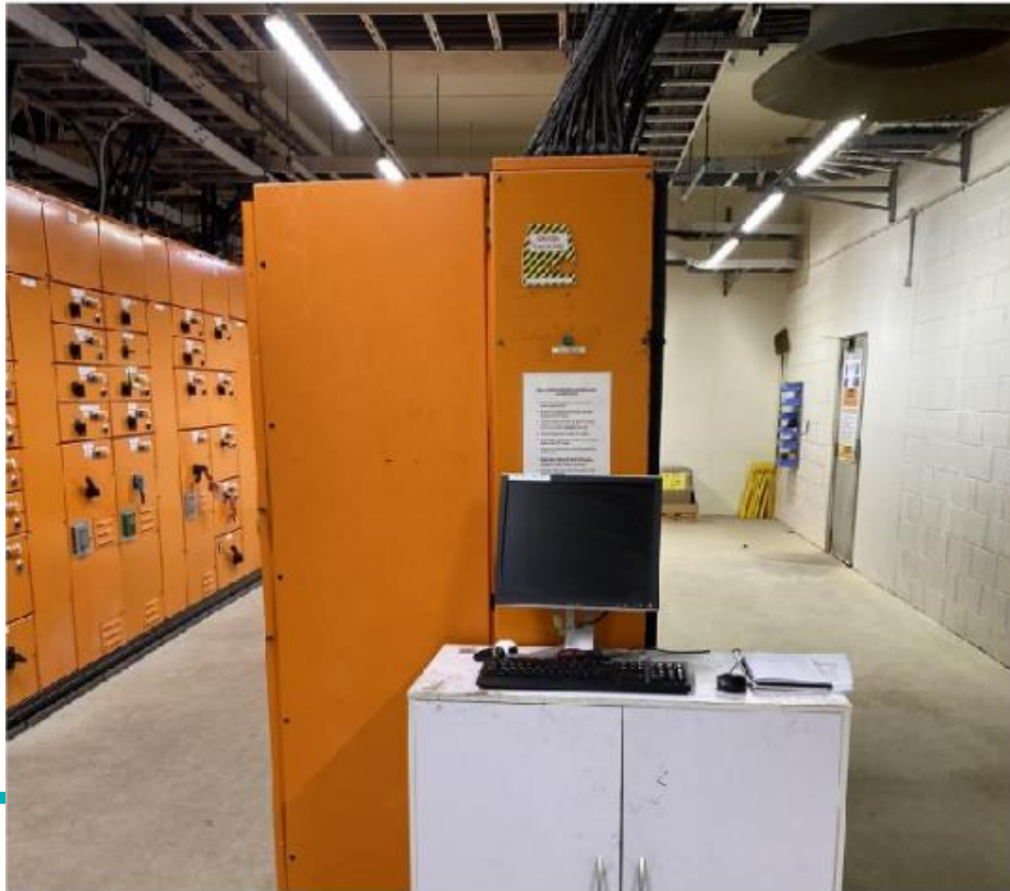
Photo of the site's Motor Control Center (MCC) units
