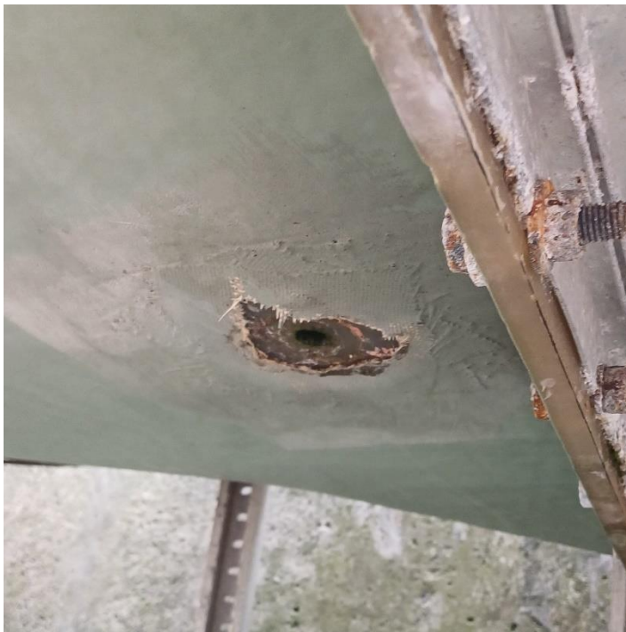
■ Figure 14: RAT and SCRT Flow Control Baffle, 23 November 2024
