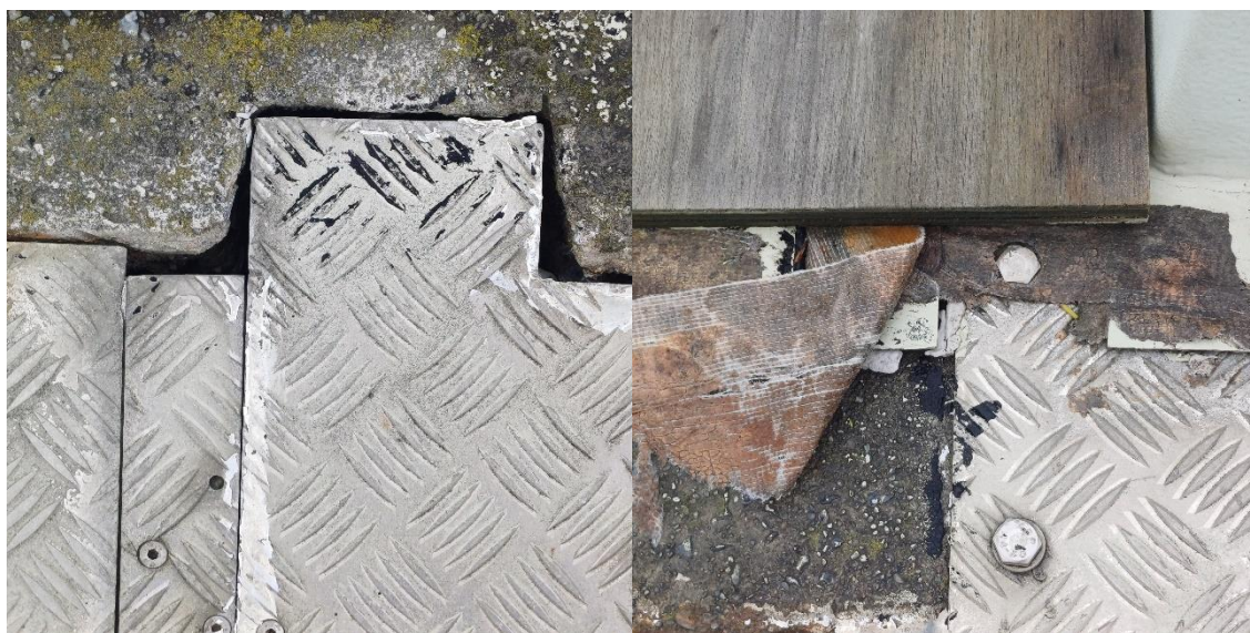
■ Figure 11: Secondary Treatment Seals, 23 November 2024
