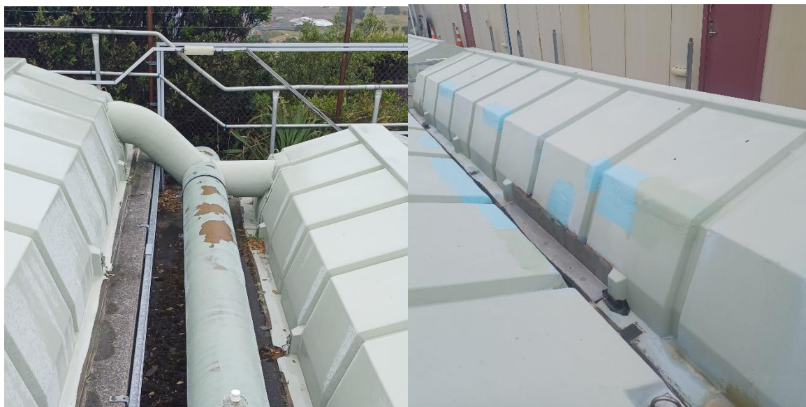
■ Figure 8: Secondary Treatment Covers & Ducting Weathering, 23 November 2024
