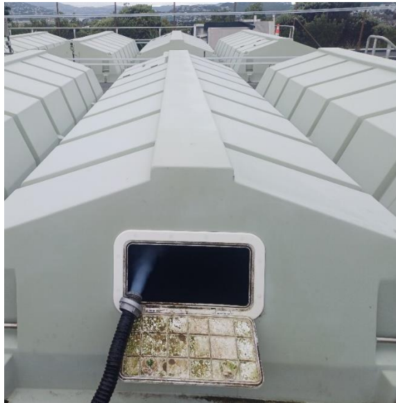
Figure 16: RATs Smoke Test, 23 November 2024
