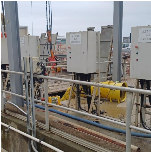
■ Figure 4: Moa Pt IPS Ventilation of Wet Well, 23 December 2024
