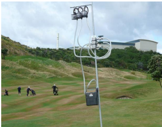
■ Figure 3: Site 3 Monitoring Equipment
