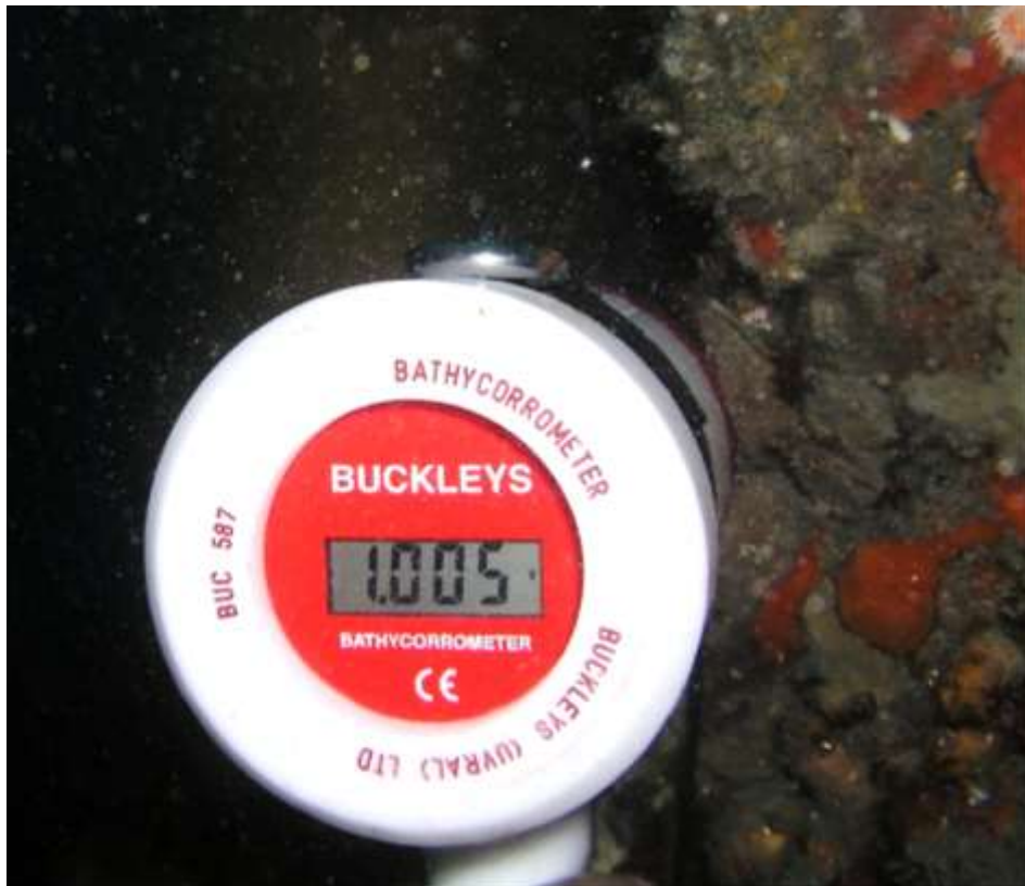
Figure 26: Cathodic Potential reading taken at Diffuser # 17
