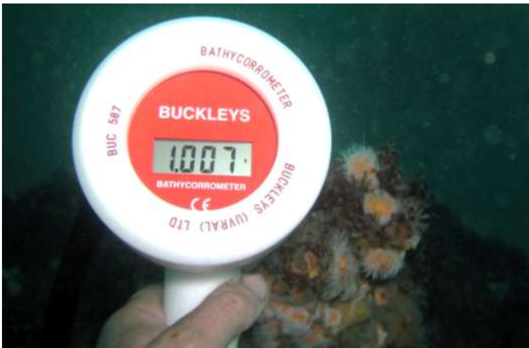
Figure 22: Cathodic Potential reading taken at Diffuser # 1
