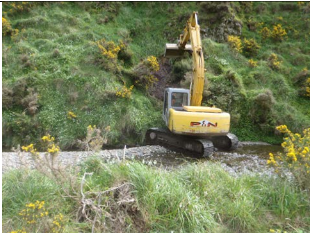
Example photo of digger working from gravel beach to expose buried leak.
