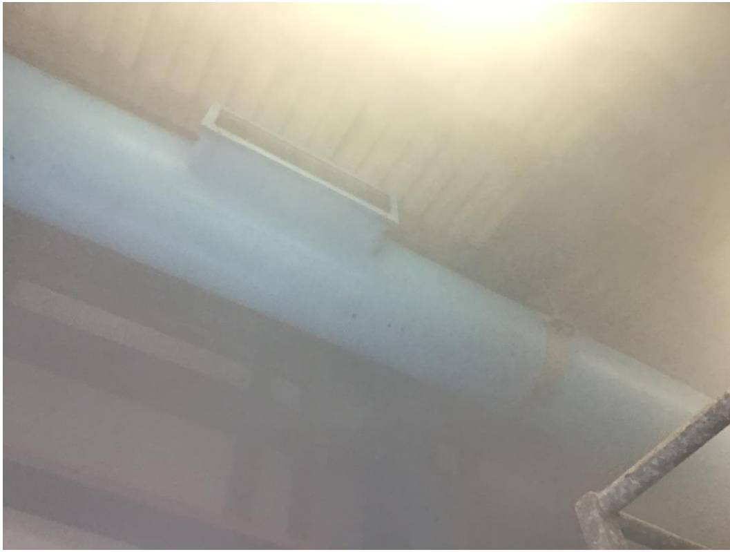
Figure 6 Demonstrates the smoke evacuating from the skip bay via the ducting to the biofilter.
