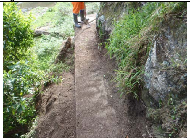
After photo of minor slip debris ontop of encased pipe.
