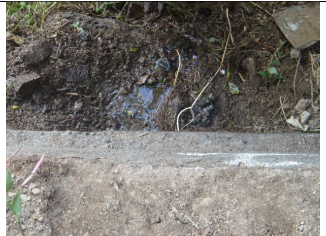
Example of minor leak found under pipeline after vegetation cleared.
