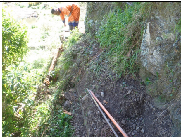
Before photo of minor slip debris ontop of encased pipe.
