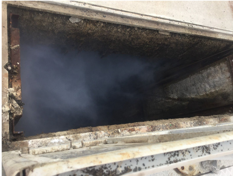
Smoke inside inlet well chamber
