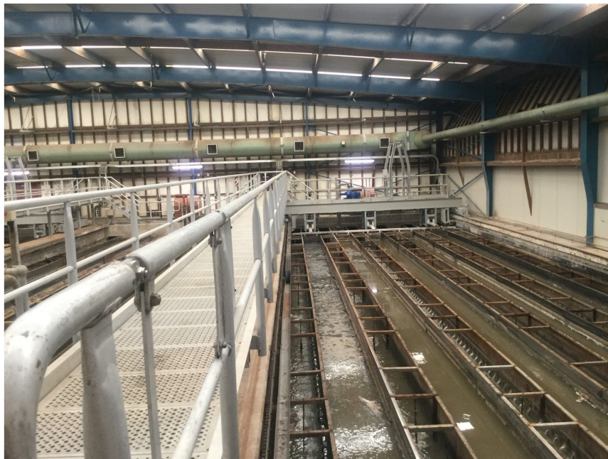
View of the primary tank area after 30minutes we turned off the machine
