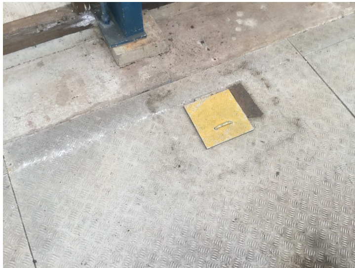
Sample hatch in MBBR common channel
