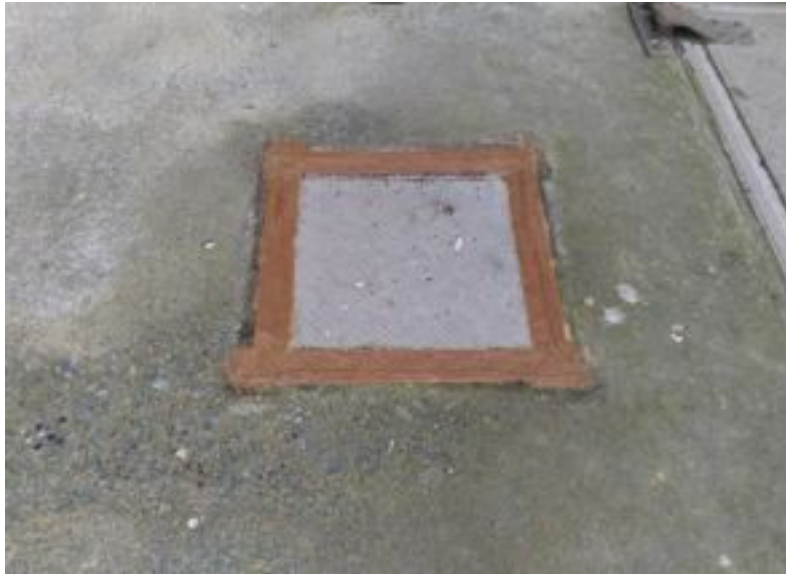
Typical seal around level sensor access hatch
