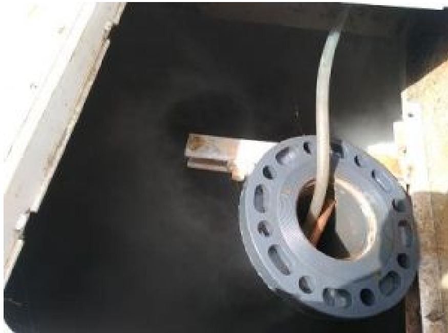
Smoke escaping from the inspection hatch once the temporary cover is removed.
