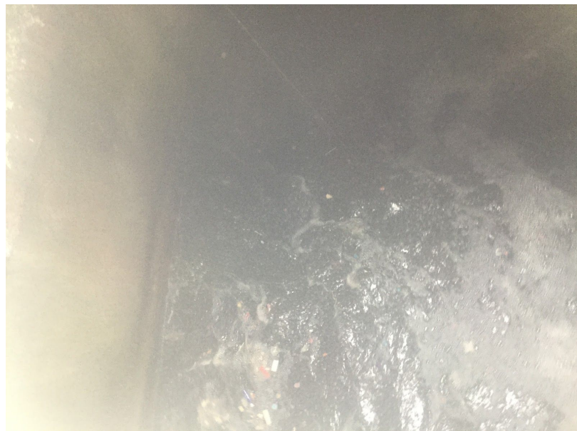
Smoke saturation in MBBR Tank
