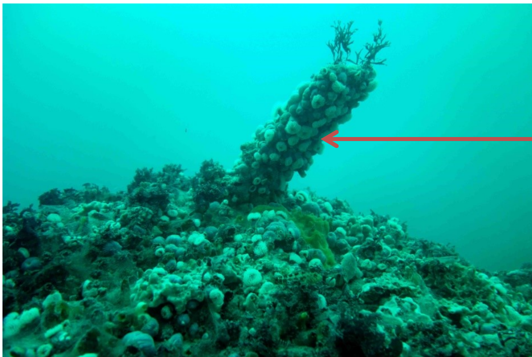
Figure 23: Diffuser # 1 (seaward southern- most diffuser) – CP test point. Readings at this position provide evidence of electrical continuity through the diffuser section
