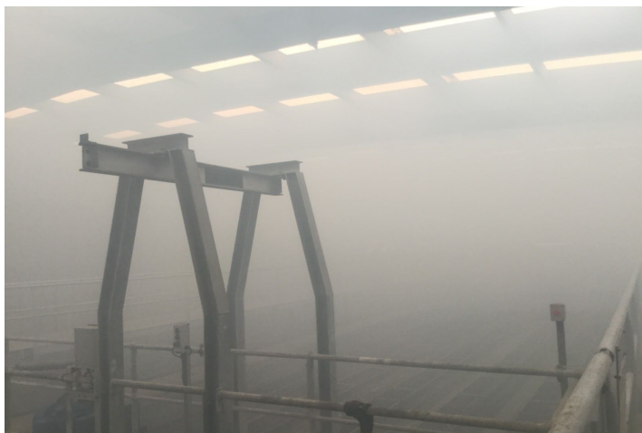
Smoke starting to build up under Primary Tank Roof
