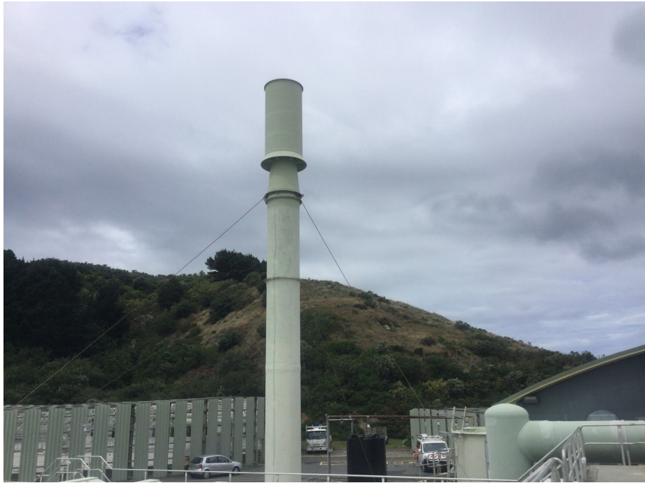
Moa Scrubber stack
