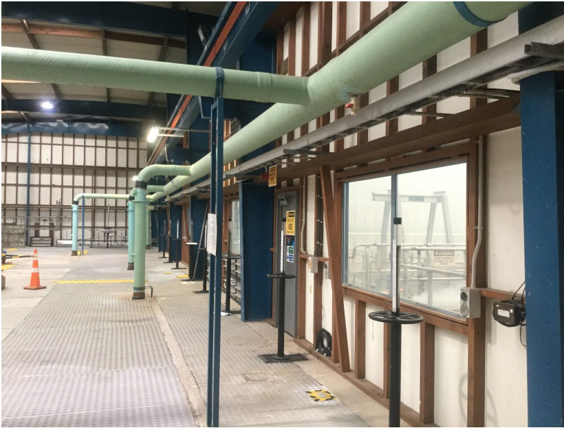
View from the step screen area
