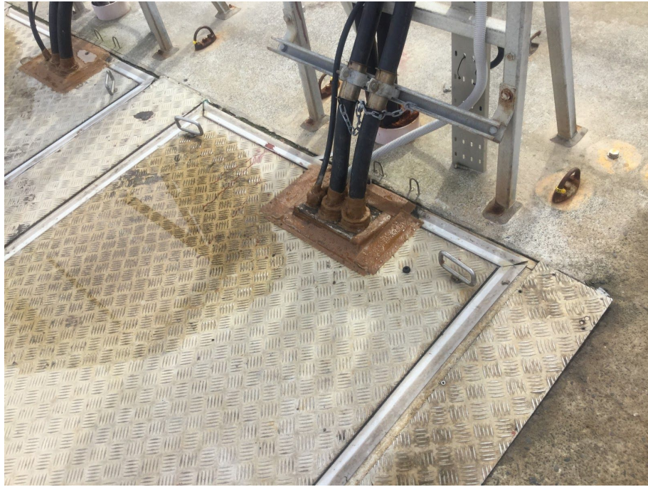
Seal around IPS Pump Cables
