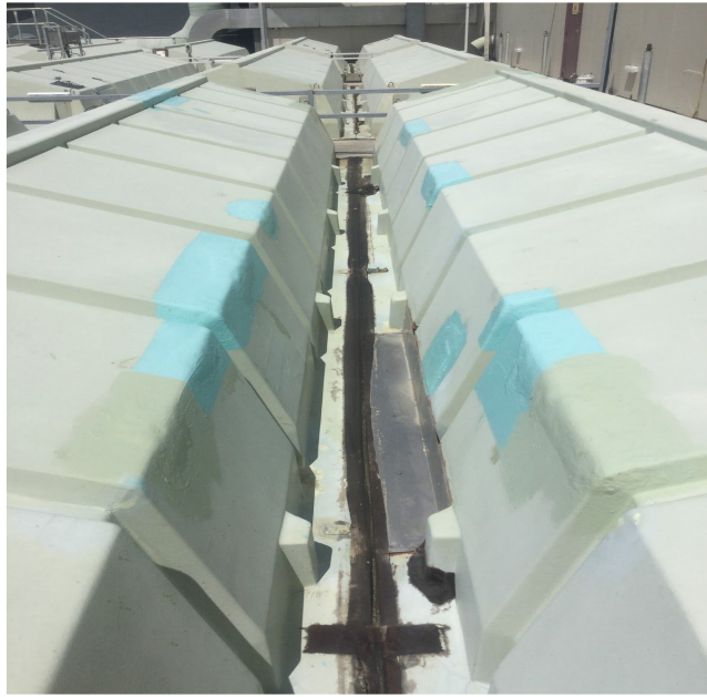
Seal between MBBR Covers
