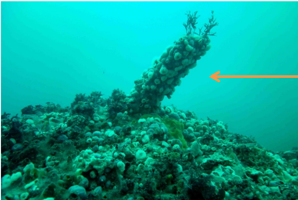
Figure 25: Diffuser # 1 (seaward southern-most diffuser) – CP test point. Readings at this position provide evidence of electrical continuity through the diffuser section
