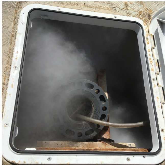
Smoke being drawn in by the vacuum inside the well once the temporary cover was removed.
