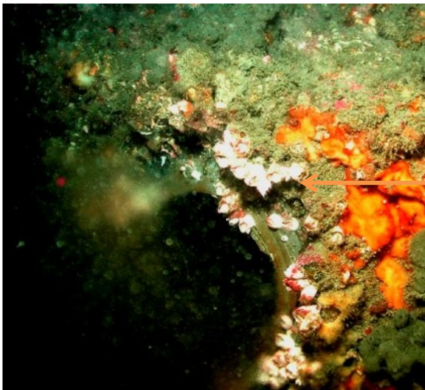
Figure 27: The steel diffuser nozzle outer flange is where the diver makes contact with the Bathykorrometer to obtain the Cathodic Potential values
