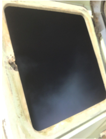
Smoke saturation in MBBR Tank
