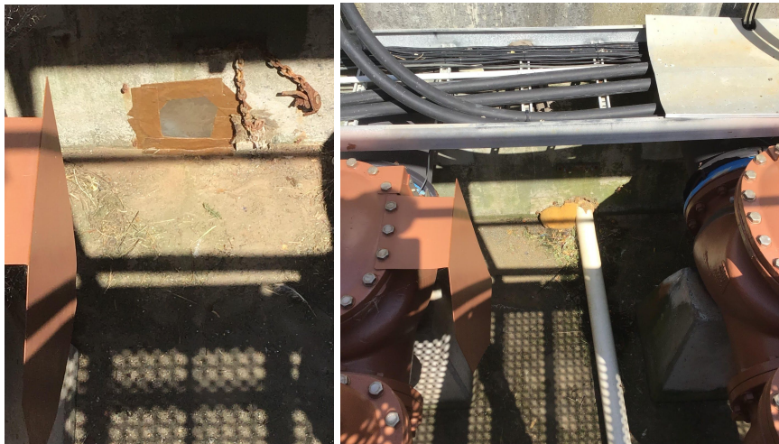
Seal around IPS Dry Well
