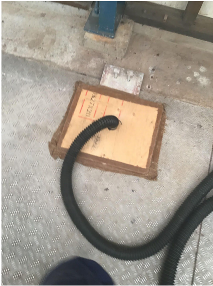
Smoke directed flooding channel to MBBR
