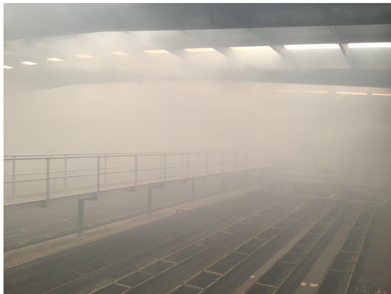
Smoke starting to build up under Primary Tank Roof
