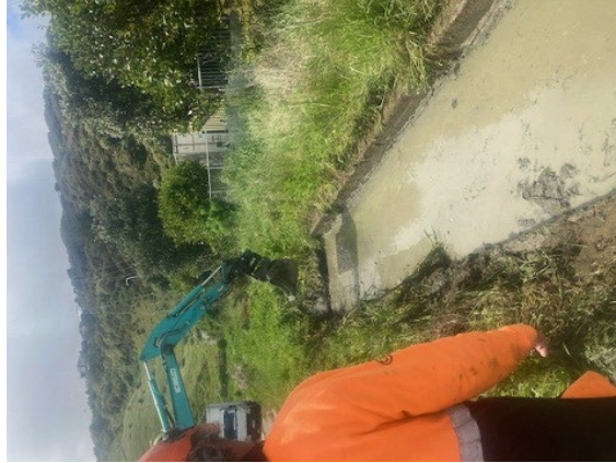
A Wellington Water crew clearing the stormwater culvert near James Street, Plimmerton
