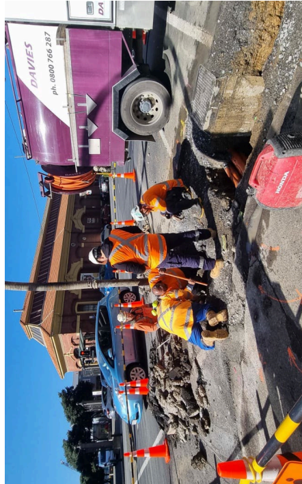
Crews busy repairing the burst water pipe on Customhouse Quay. Photo: RNZ/Krystal Gibbens
