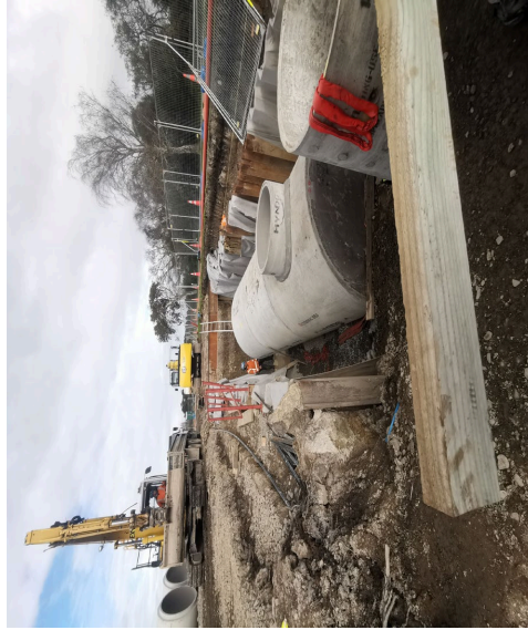
Donald St Pump Station in Featherston
