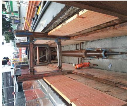
New section of pipe being installed as part of the Taranaki Street Rising Main Project in central Wellington.
