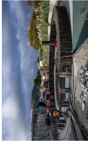
Sections of the new wastewater storage tank in Porirua being built. Once completed the tank will hold wastewater during times of heavy rain to reduce overflows into the environment.
