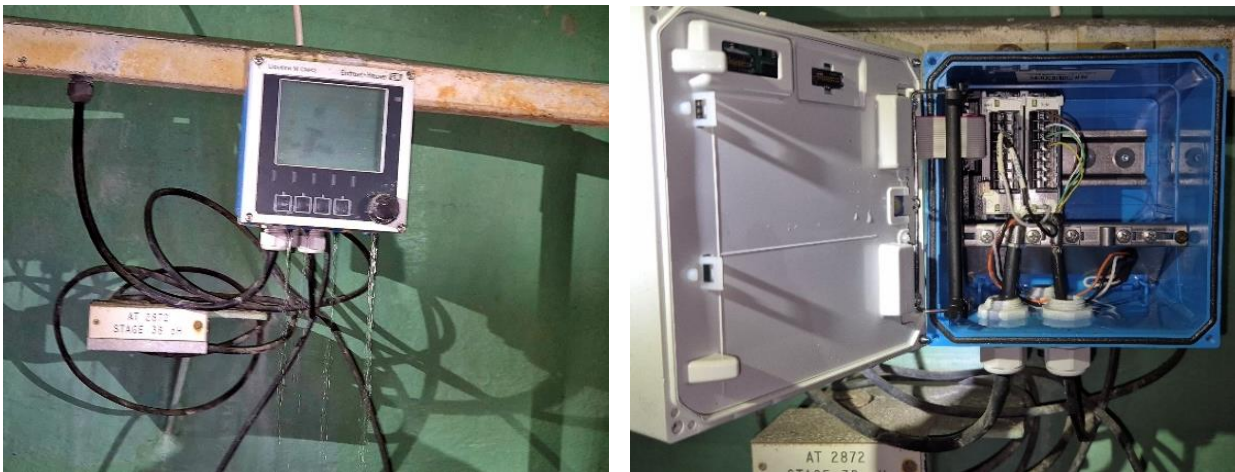
Figure 12: Scrubber analyser transmitter (L and R)
