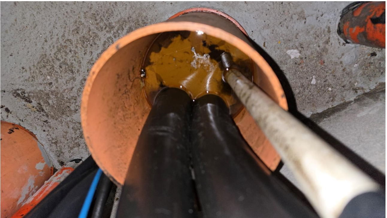
Figure 66: Blower motor cables ducting with liquid still inside.
