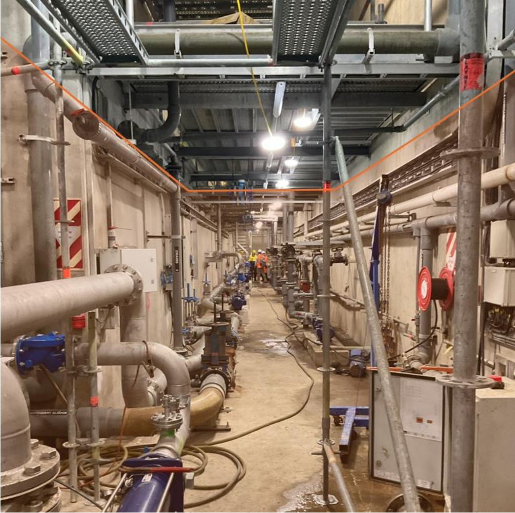
Figure 23: Primary Sludge Pumps Technical Gallery indication of the approximate level to which assets were submerged
