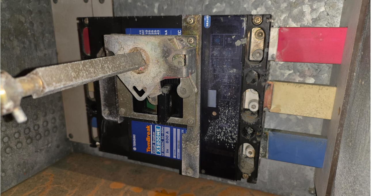
Figure 76: Affected MCC Cells, Isolators
