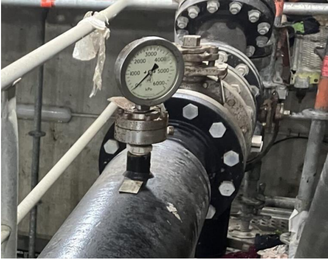
Figure 45: Sludge transport pressure gauge
