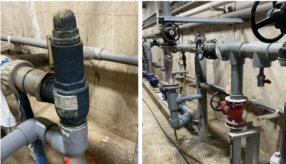
Figure 30: Primary Sludge Pump pressure relief valve (L) and Primary Sludge pipework and valves (R)
