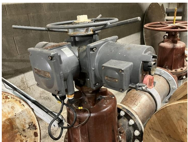
Figure 57: WAS pipework in service gallery
