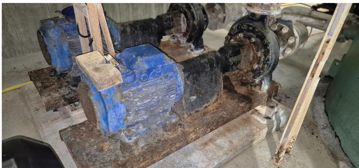
Figure 17: Odour Scrubber Recirculation Pump (Stage 3B)
