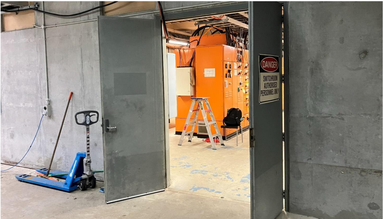
Figure 53: Location of pallet truck in service gallery
