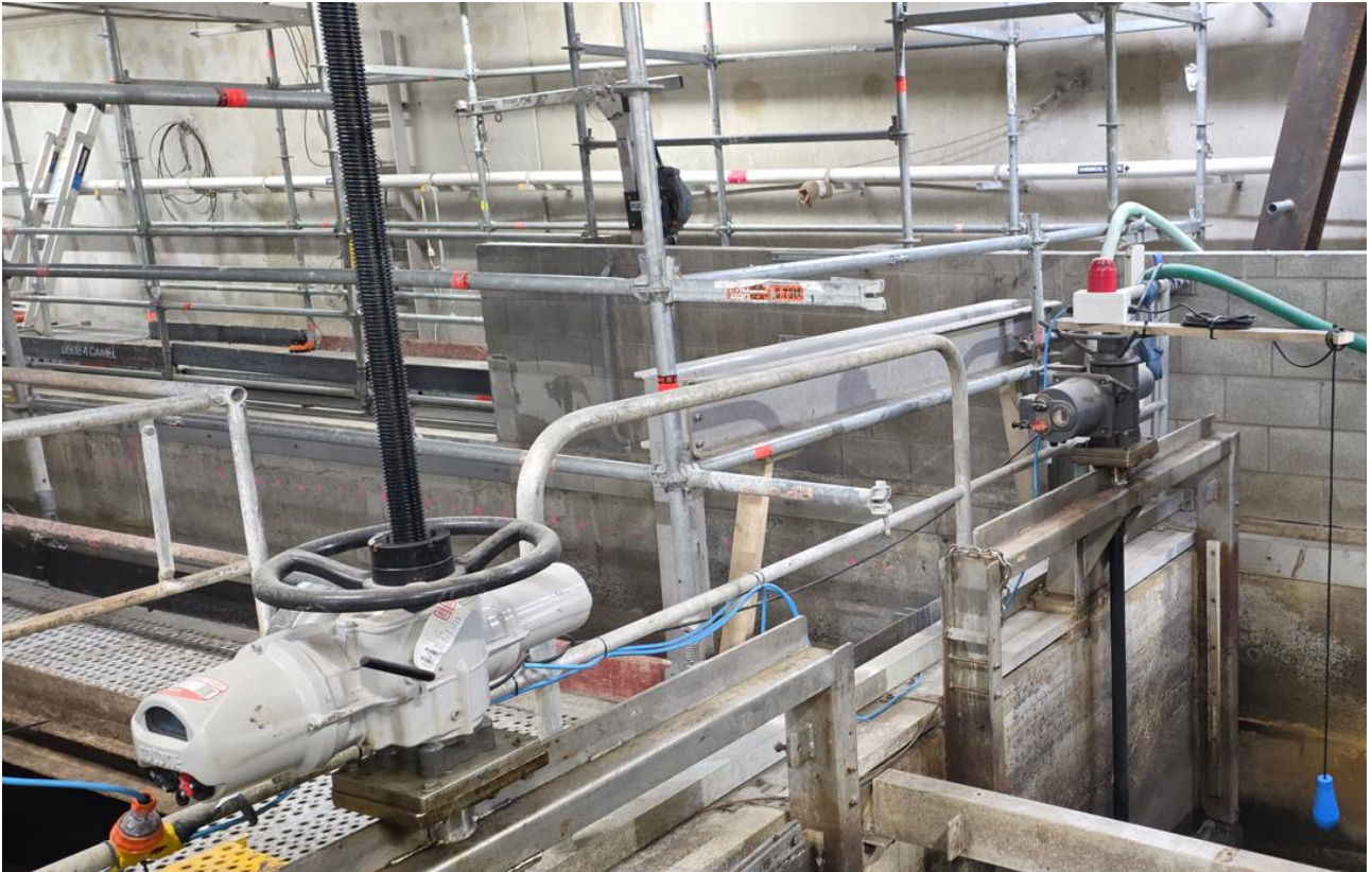
Figure 94: UV System Actuated Penstock Valves
