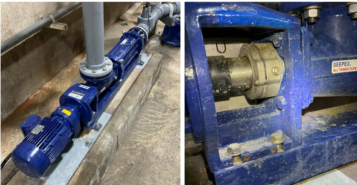
Figure 27: Primary Sludge Pump 6 (L) and pump shaft and seal (R)
