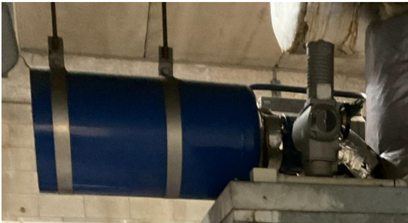
Figure 60: Blower Exhaust Air Silencer
