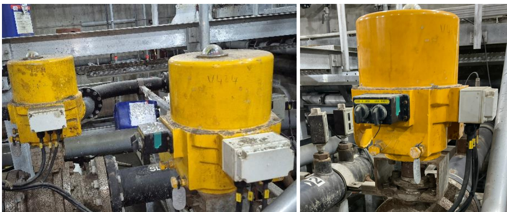
Figure 50: Sludge Pipeline Actuated Valves
