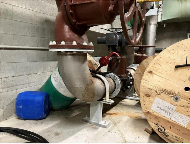
Figure 56: WAS pipework in service gallery
