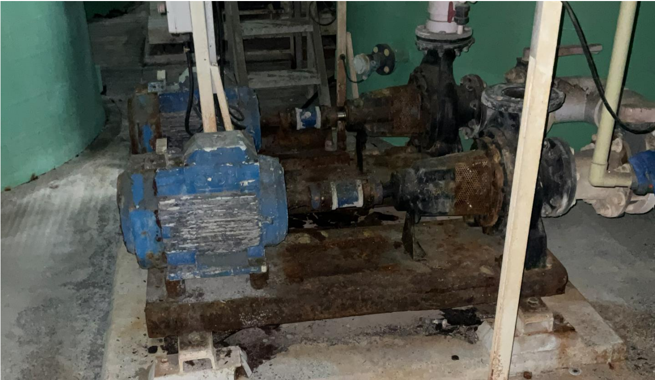
Figure 19: Odour Scrubber Recirculation Pump (Stage 1B)
