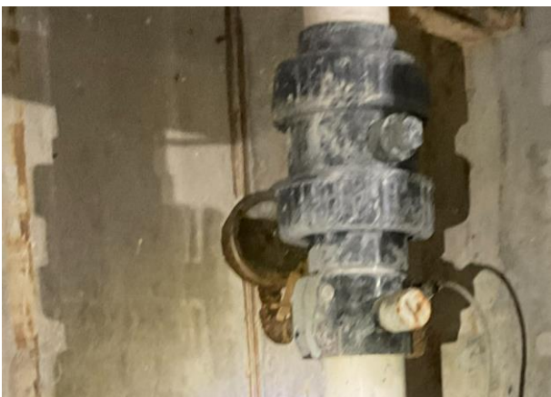
Figure 7: Neutralisation system pressure indicator in poor condition
