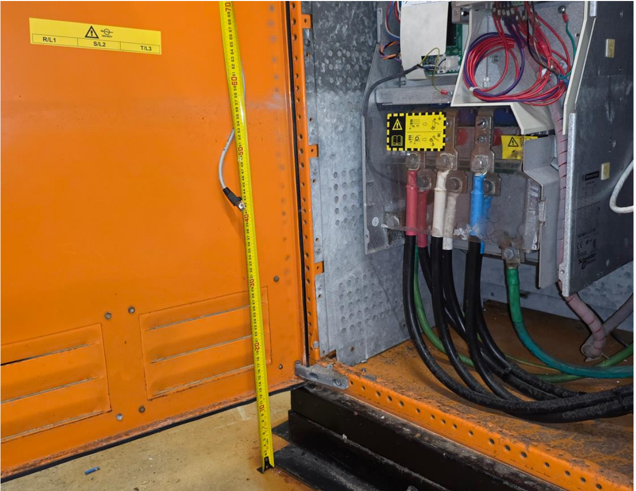
Figure 74: Waterline height and VSD terminals
