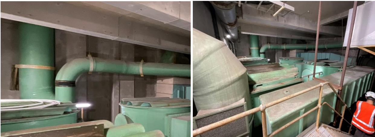
Figure 6: Foul Air Ducting
