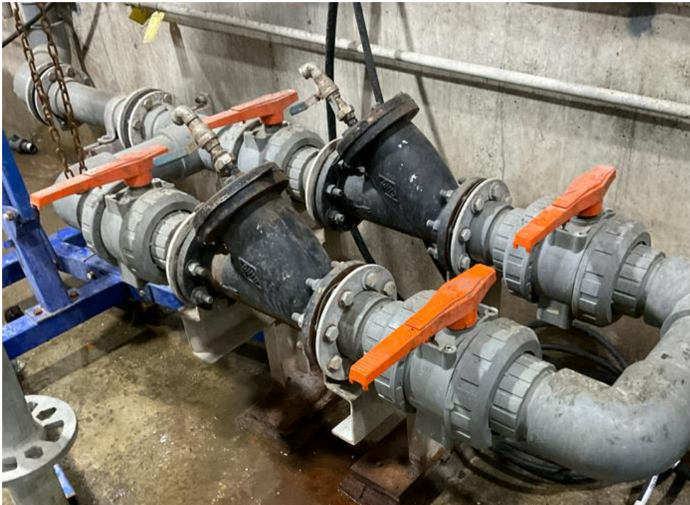
Figure 33: RE Wash Water strainers and pipework
