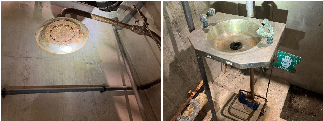
Figure 20: Safety shower and eyewash station
