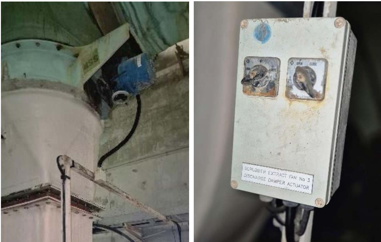
Figure 13: Actuated odour control damper (L) and local control station (R)
