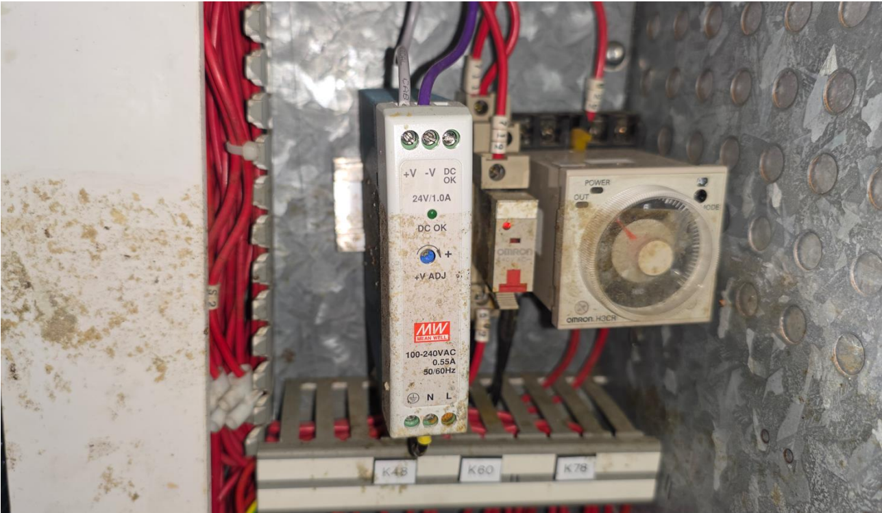
Figure 79: Electronics partially submerged
