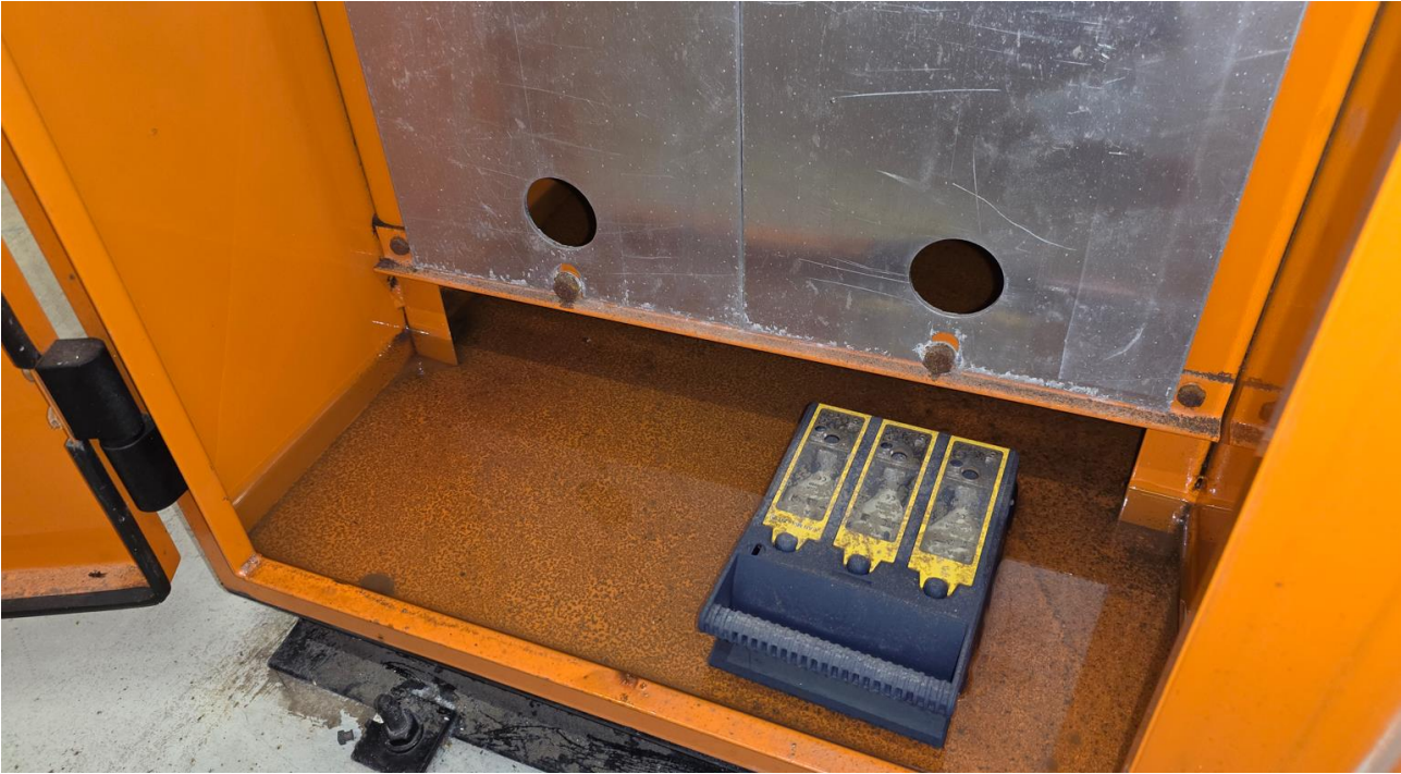
Figure 81: Residual wastewater in Power Factor Correction panels
