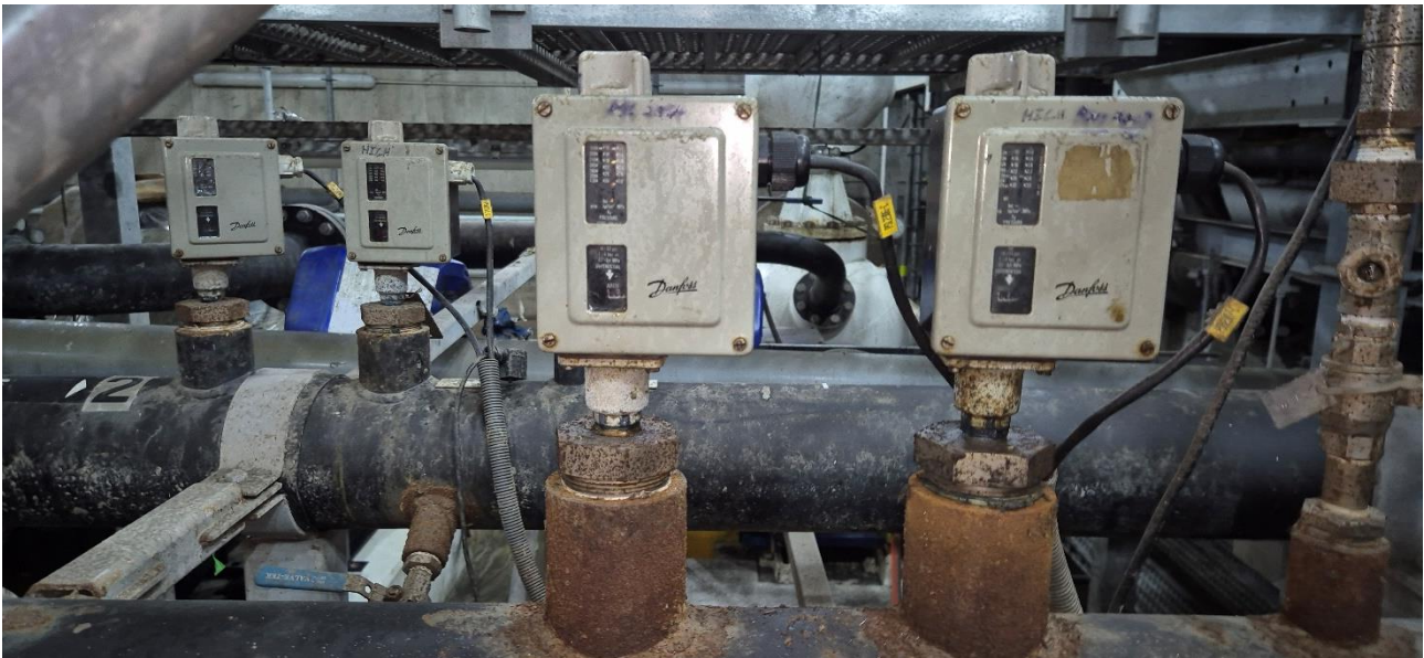
Figure 44: Sludge transport pressure switches and gauges
