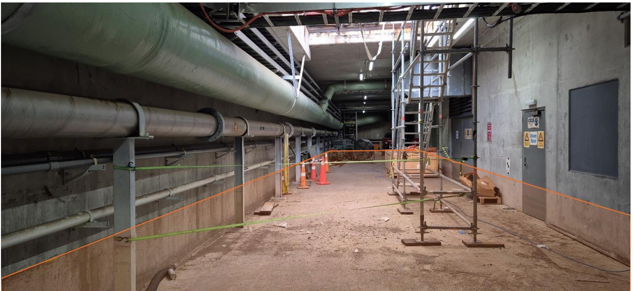
Figure 52: Service Gallery indication of the approximate level to which assets were submerged
