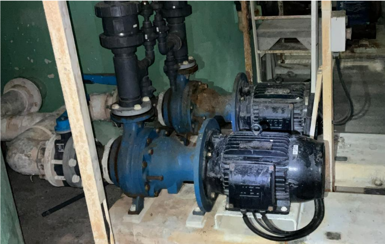
Figure 18: Odour Scrubber Recirculation Pump (Stage 2A)
