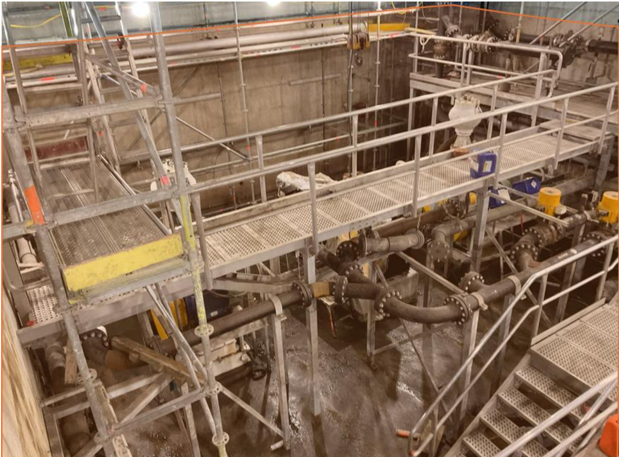
Figure 42: Sludge Transport Pumps Chamber indication of the approximate level to which assets were submerged
