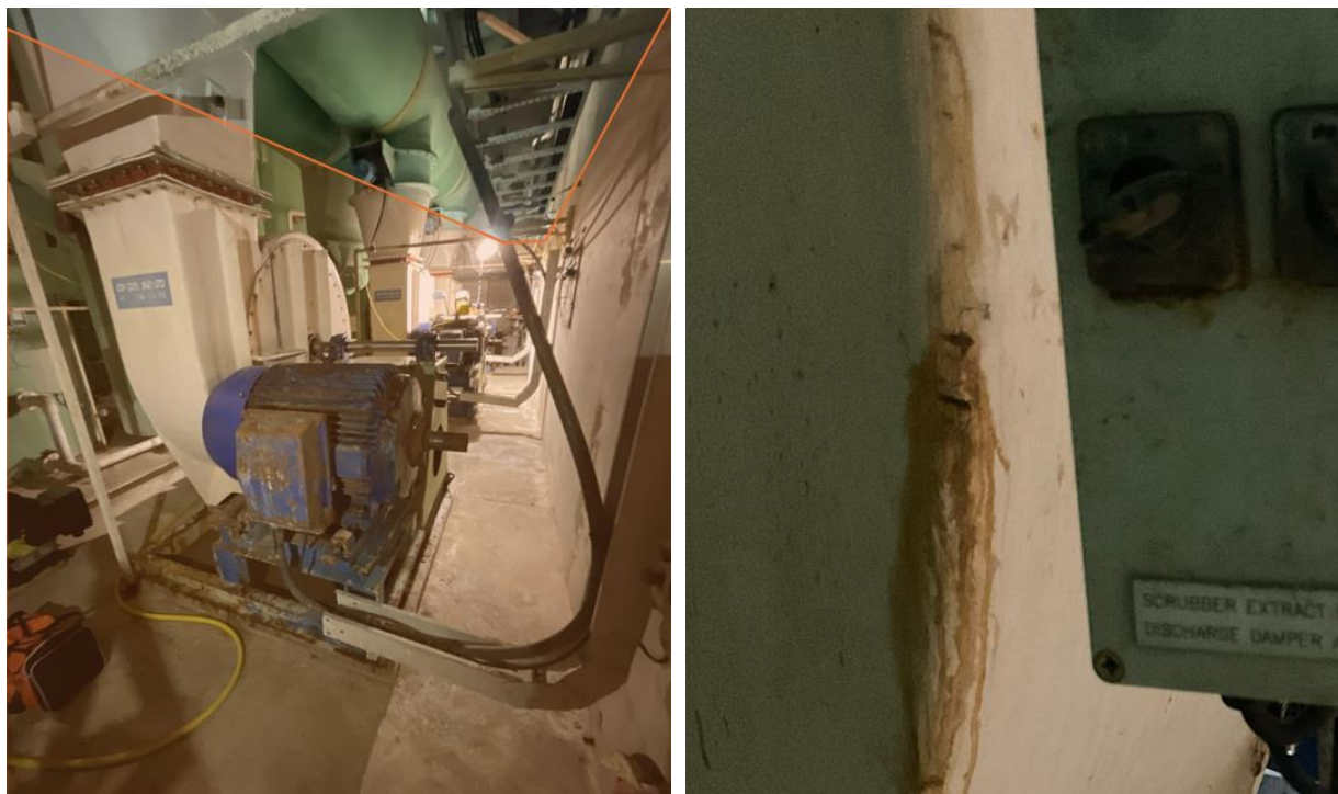
Figure 10: Odour control extraction fans indicative level of submergence (L) and Scrubber Extraction Fan 2 housing damage where ingress is likely to occur (R)
