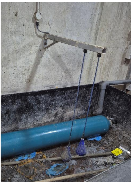
Figure 31: 25-T004 Primary Sludge Pump Relief Tank level switches and terminal box
