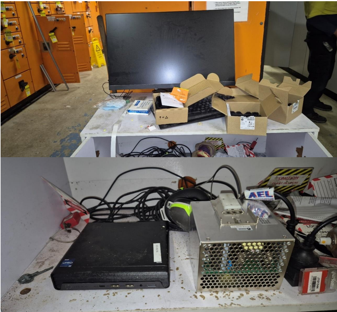
Figure 87: Switchroom SCADA client PC, power supply and monitor
