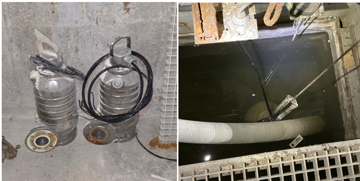
Figure 8: Neutralisation Discharge Pumps (L) and installed Neutralisation Discharge Pump in the well (R)
