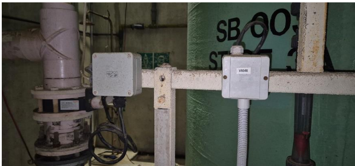
Figure 16: Odour scrubber piping and valves (electrical connection boxes)
