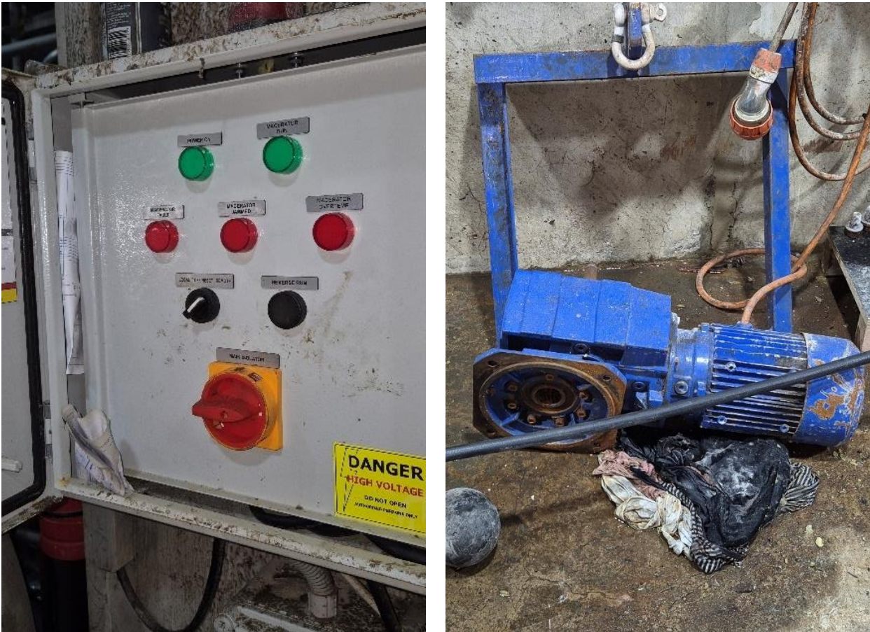
Figure 39: Mono Muncher electrical control panel (L) and gearmotor (R)
