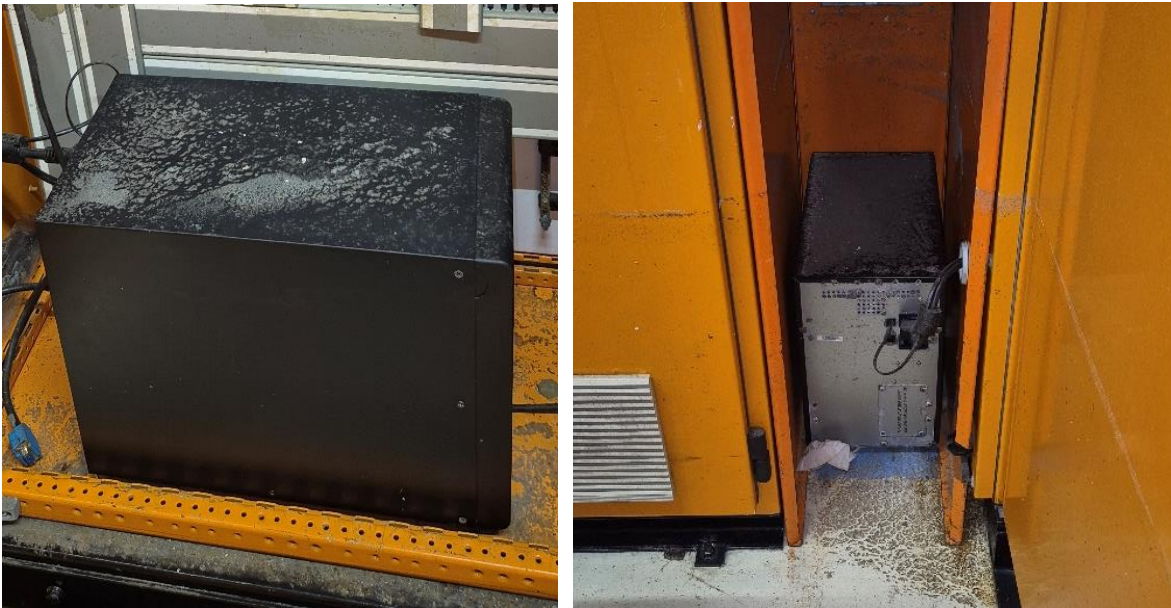
Figure 86: PLC UPS (L) and Battery Pack (R)
