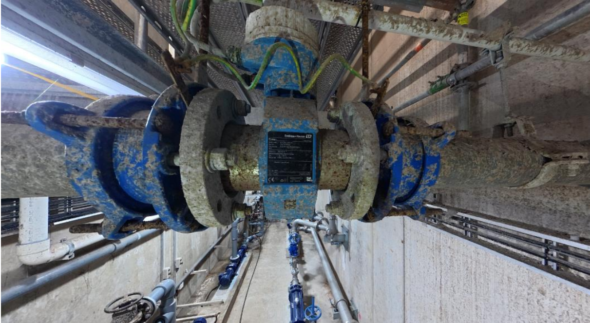
Figure 25: Primary sludge flow meter and flow transmitter.
