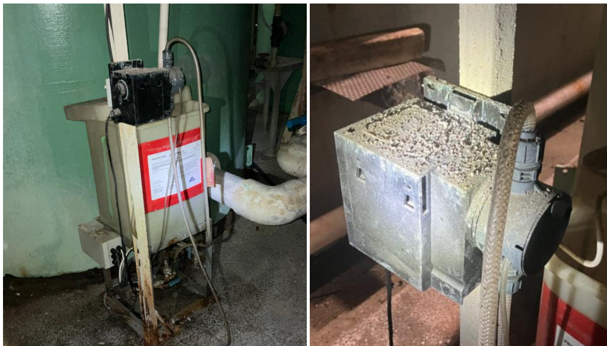
Figure 5: Anti Scalant Dosing System (L) and Anti Scalant Dosing Pump (R)
