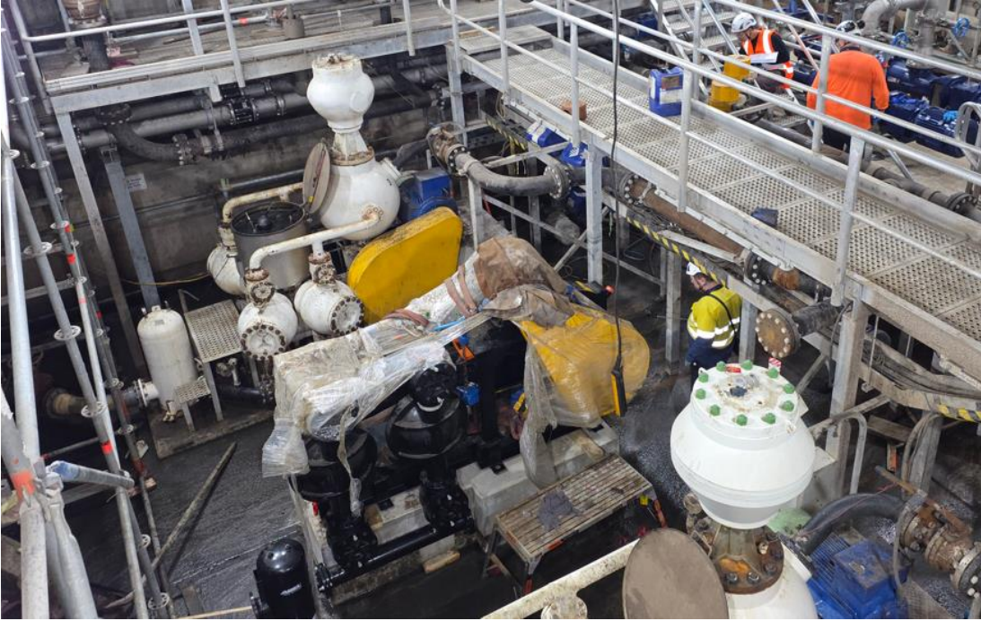
Figure 47: Sludge Transport Pumps
