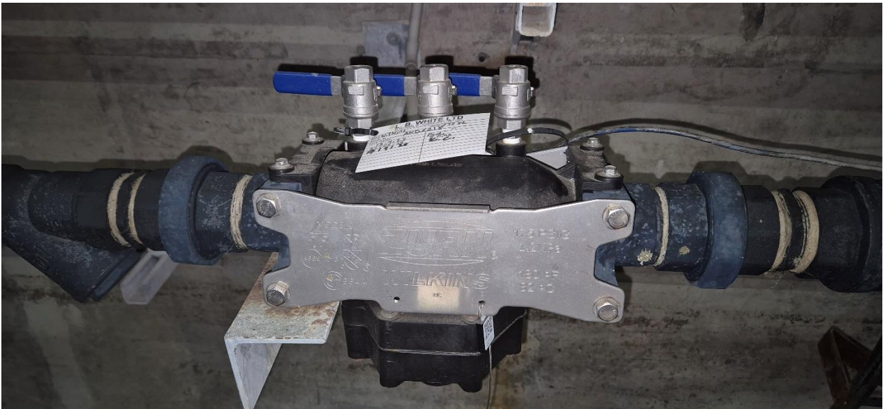
Figure 54: RPZ Backflow Preventer in Service Gallery
