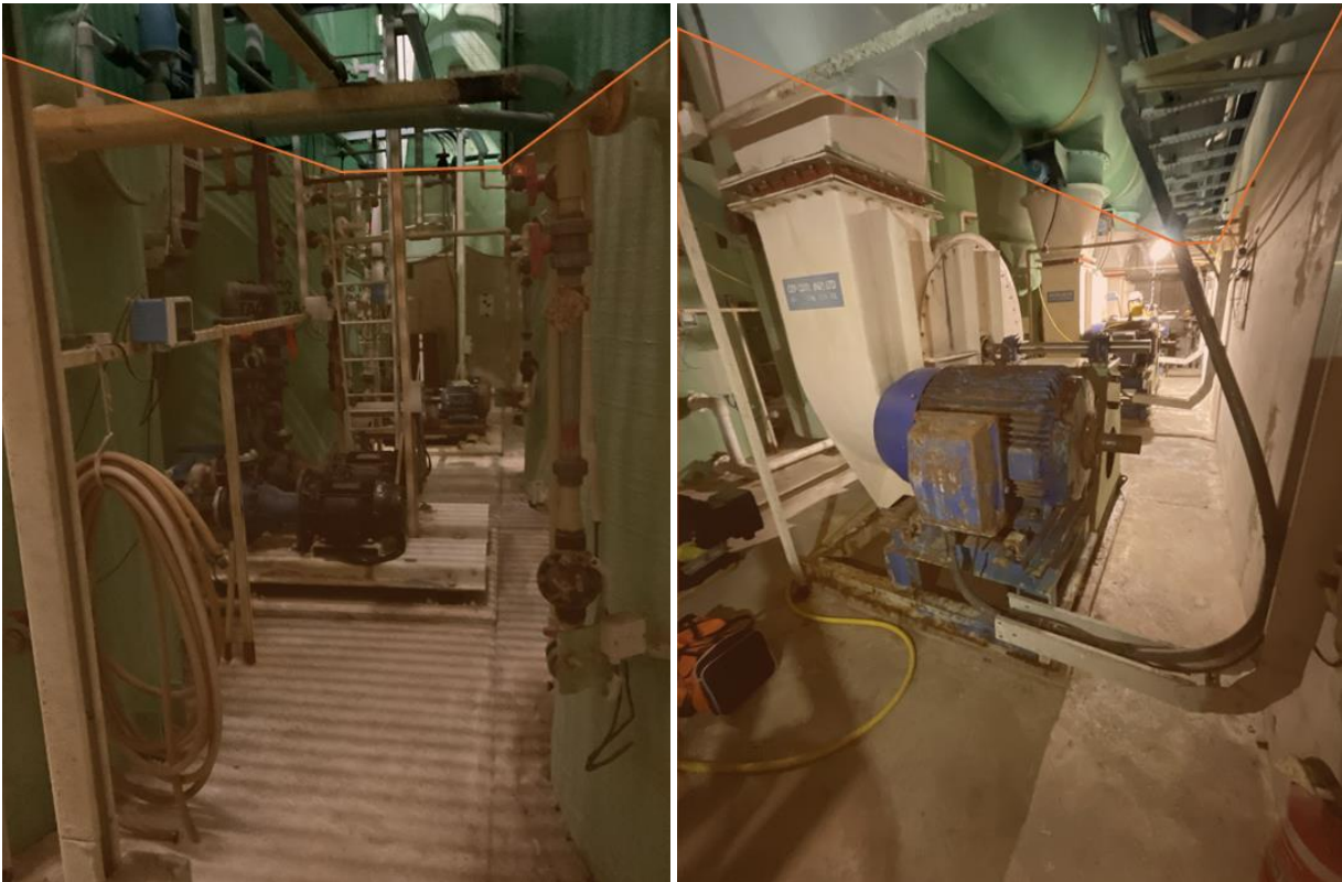
Figure 4: Odour Control Room indication of the approximate level to which assets were submerged (Scrubber recirculation pumps, (L), Scrubber extraction fans (R))
