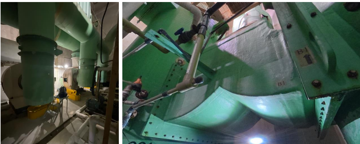
Figure 14: Odour control ducting
