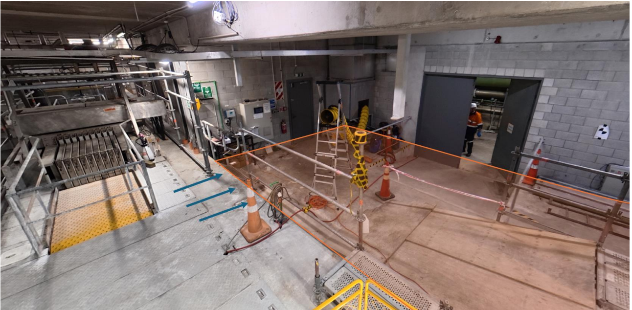
Figure 89: UV Room indication of the approximate level to which assets were submerged
