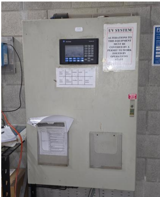
Figure 92: UV Control Panel
