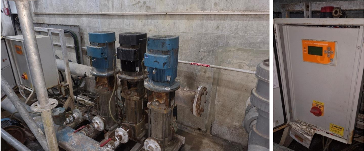
Figure 34: RE Wash Water pumpset (L) and controller (R)
