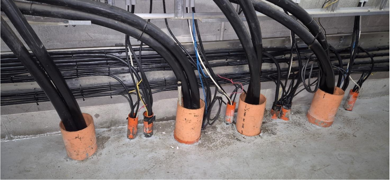
Figure 65: Blower motor cables, power cables and control cables through ducting in floor to individual blowers
