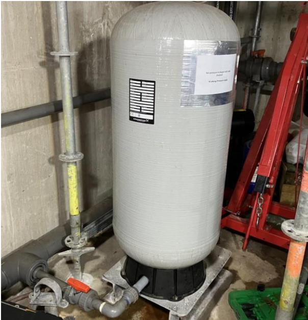
Figure 35: RE Wash Water Accumulator Tank
