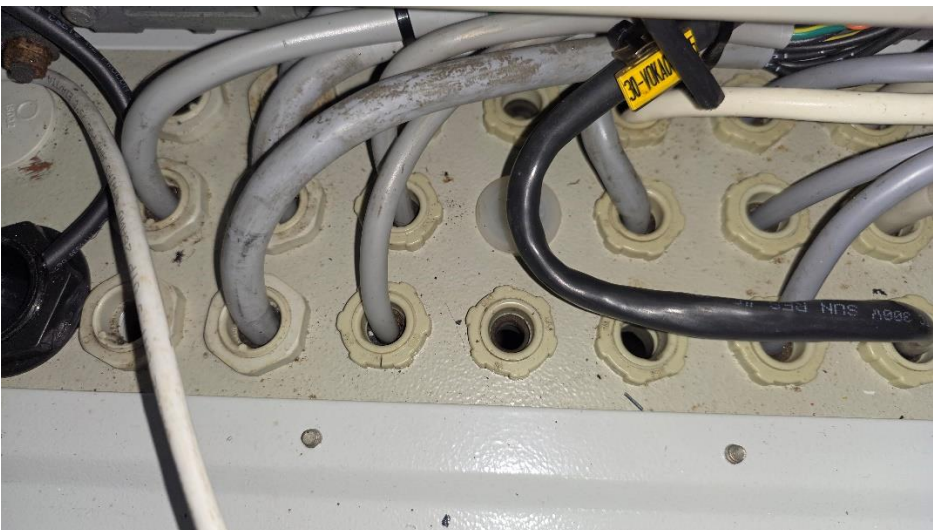
Figure 64: Blower control panel showing unsealed gland holes.
