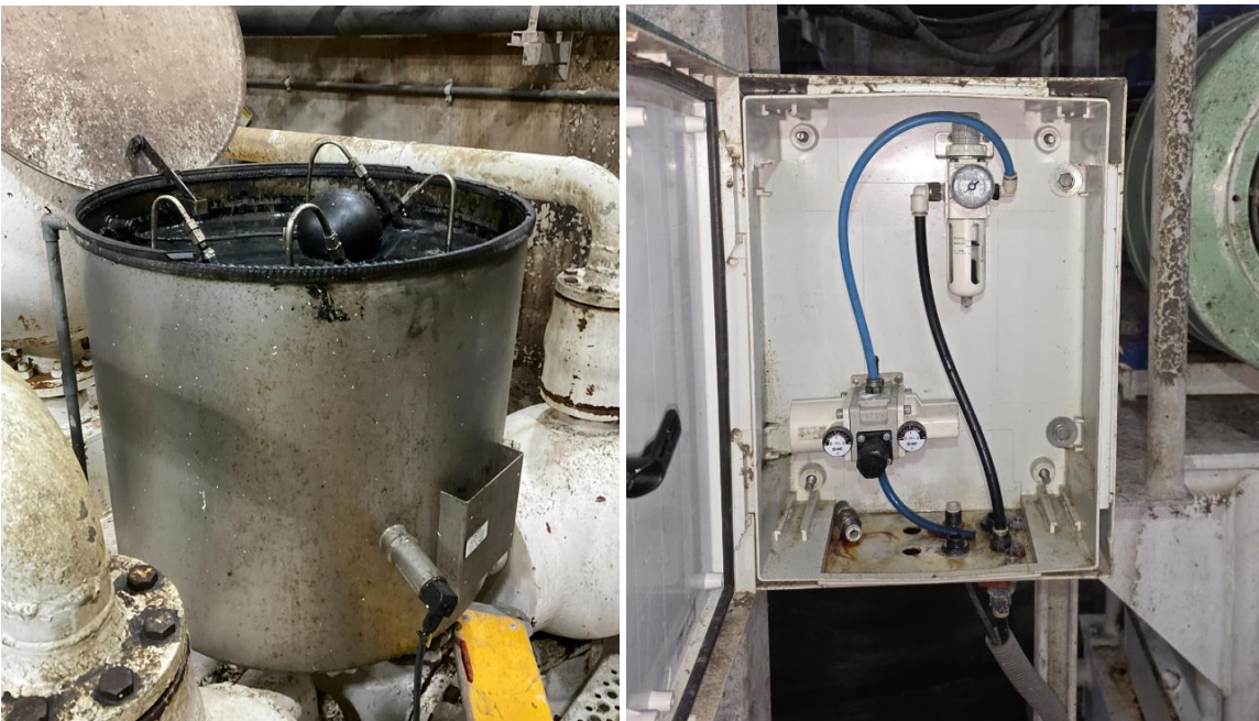
Figure 48: Sludge Transport Pump water storage tank (L). Compressed air system regulator and solenoid. (R)
