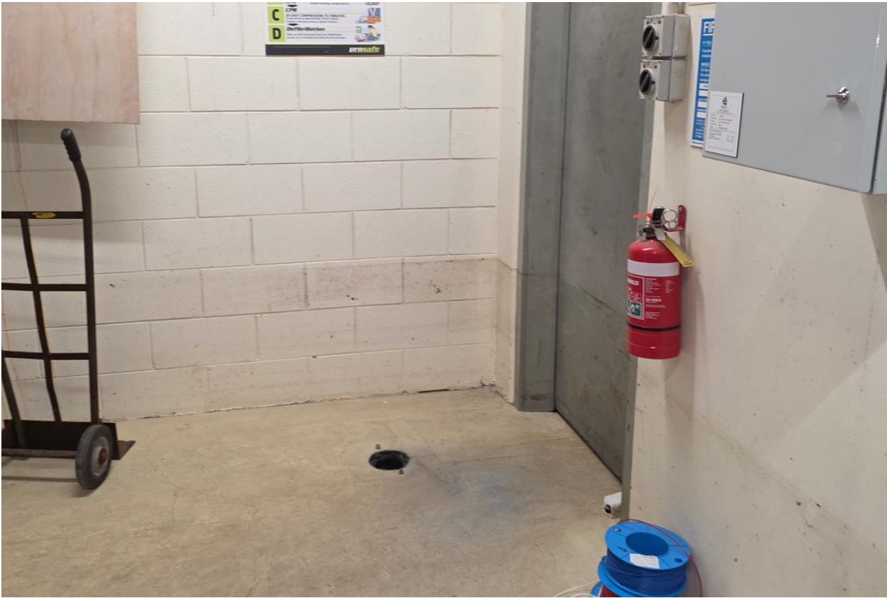
Figure 71: Waterline mark in Switch Room
