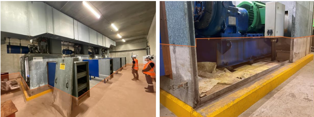
Figure 59: Blower Room indication of the approximate level to which assets were submerged - Blower room water level (L) and Blower 1 base frame water level (R)
