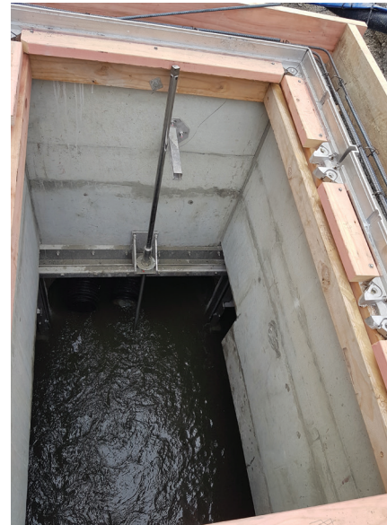
The enlarged chamber lid and penstock in operation. Due to space restrictions above the chamber, the penstock has to close upwards rather than downwards as they typically do when shutting off water.
