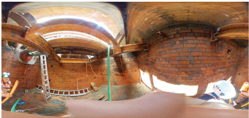
Temporary supports were installed to support the chamber roof during the upgrade.
