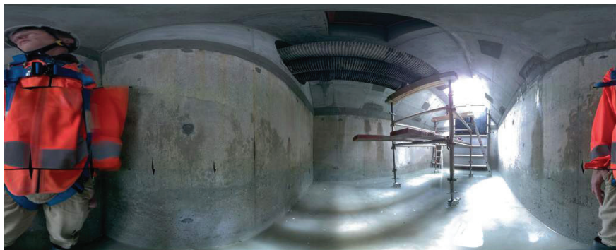
The chamber after seismic strengthening and functional improvements. It will need to be cleared of gravel once every very two or three years now, rather than annually, and will be much safer for workers.
