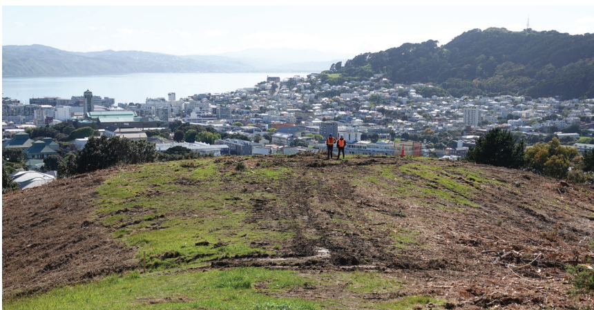
The new Omāroro reservoir site in Prince of Wales Park in the Town Belt. Lizards living in the area are being rehomed.
