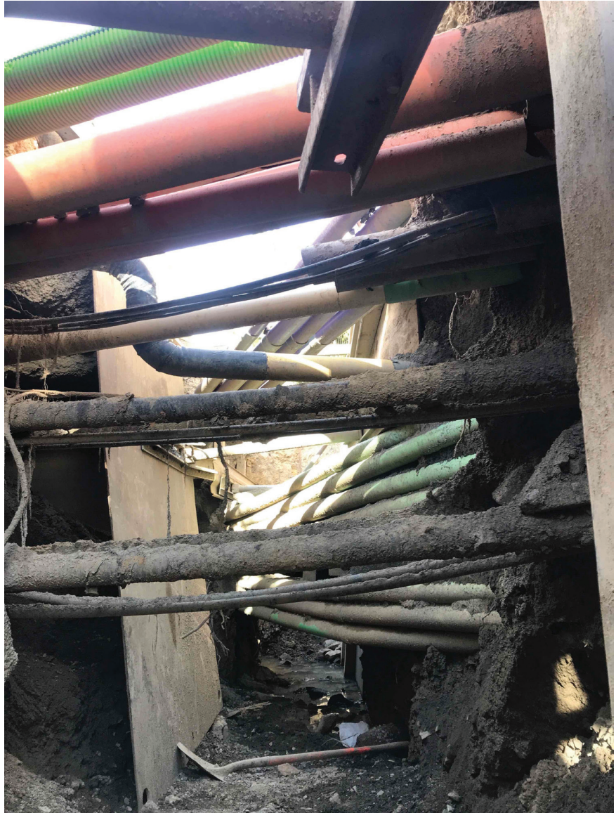
Multiple underground services are one of the complicating factors in the area.
