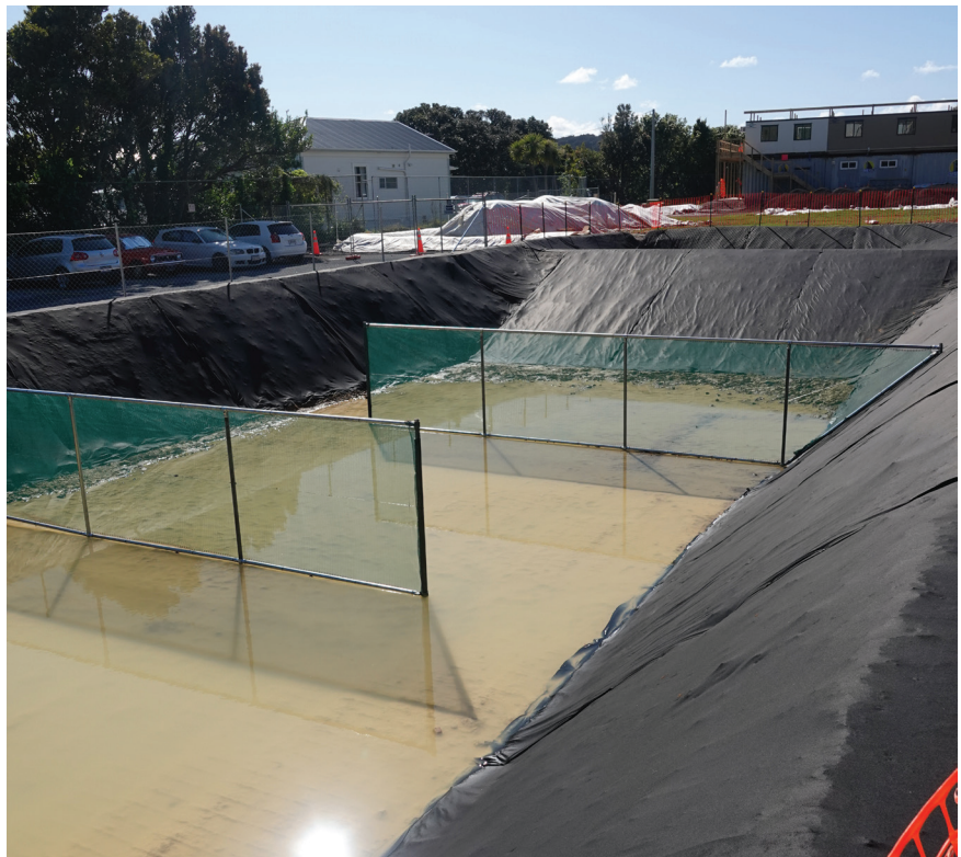
The upper field sediment pond shown here is one of two ponds that will capture runoff from the excavation. Once sediment has settled, the water collected will be used for dust control on site.
