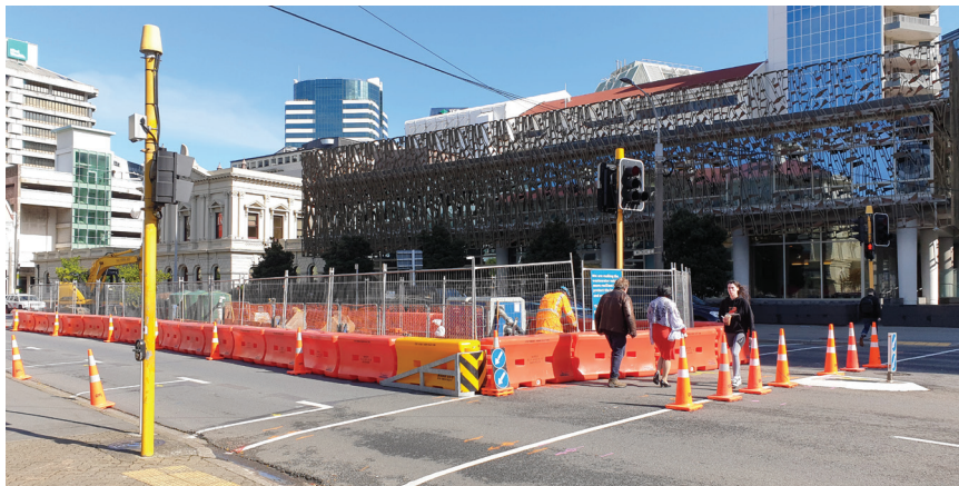
The site of the launch pit in Whitmore Street for the pipe-ramming operation beneath the busy Lambton Quay intersection.
