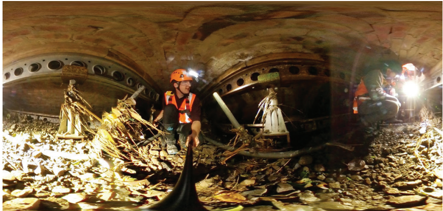
The 1930s Aro St stormwater chamber full of gravel prior to its annual clean out and the upgrade carried out by Connect Water.
