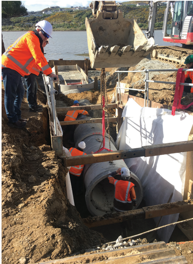
The wetland will catch the first flush of stormwater events, which carry high levels of contaminants, particularly in run-off from roads. This by-pass main, due to be completed in March 2021, will divert remaining high volume flows away from the wetland to protect it from damage and potentially overflowing.
