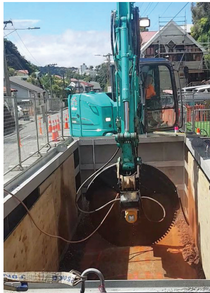
The first 'keyhole' being cut into the brick arched chamber roof. The entire roof could not be removed because of service lines in the area.
