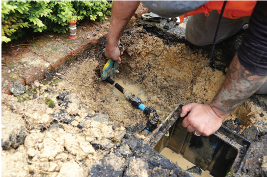
This time the fault was a pinhole leak in the pipe. The offending section was removed and replaced with a plastic fitting.
