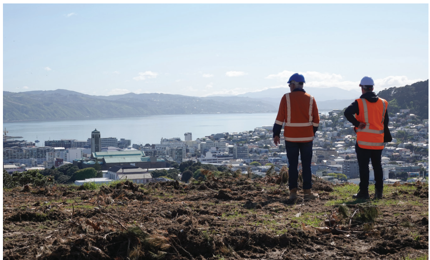
It's a great site! The new reservoir will be buried here so the park can remain a green space for the public.
