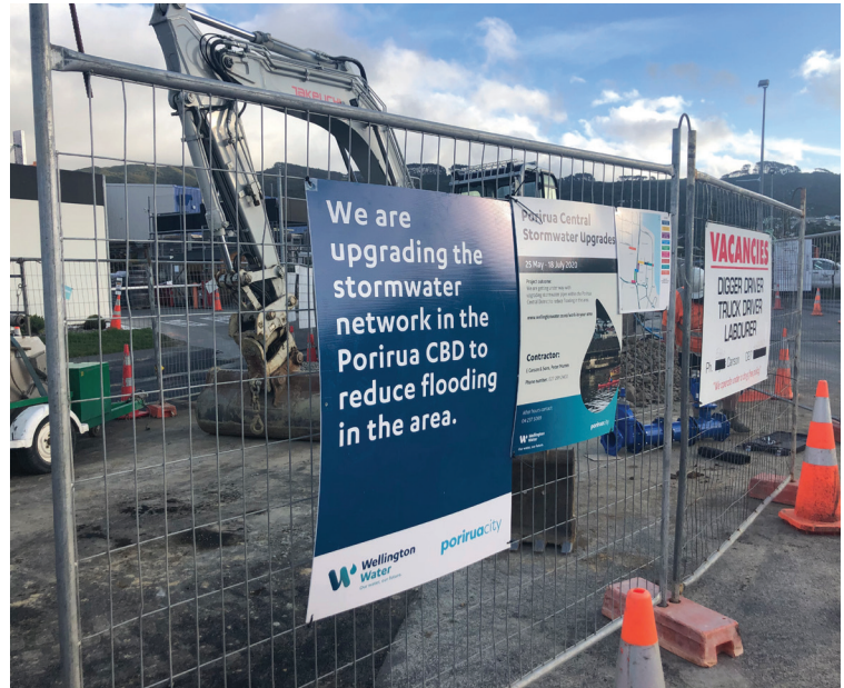
A number of projects are underway to improve stormwater management in Porirua.
