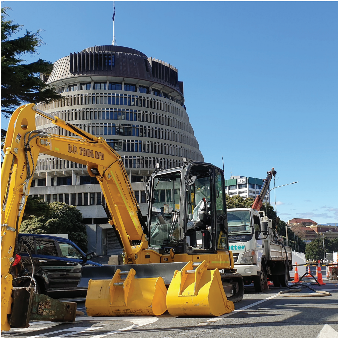
A new wastewater main is being installed in an area with heavy traffic and pedestrian flows.
