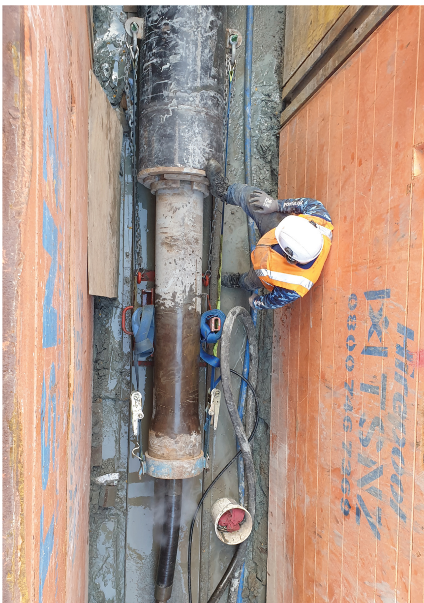
Pipe-ramming in process in Whitmore Street. This trenchless technique avoided at least four weeks of interruption to traffic and pedestrians.
