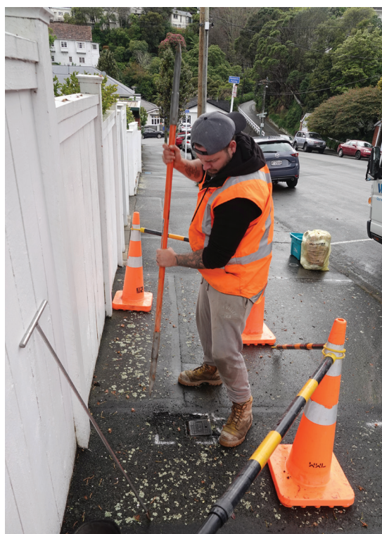
Using a hand tool to break up the pavement is much quieter for local residents.
