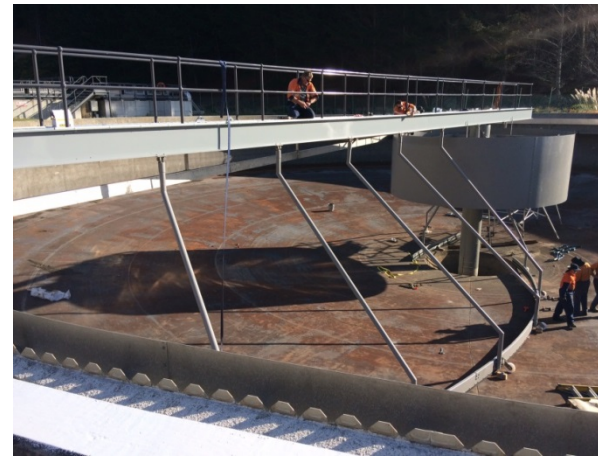
A new rotating bridge and scraper arm is installed in one of the clarifier tanks at Porirua Wastewater treatment Plant.
