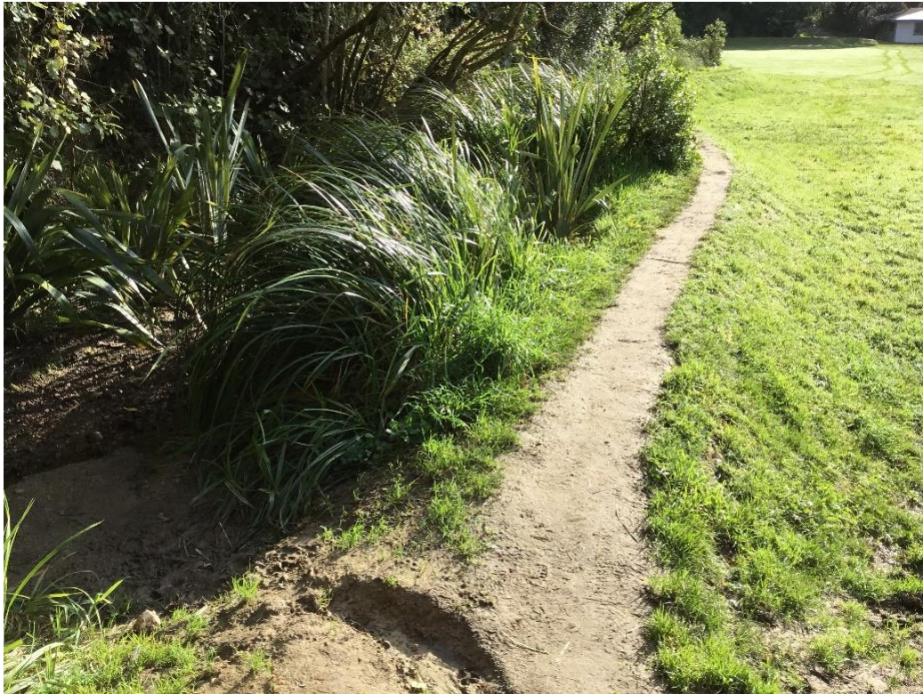
Figure 6a – Papawai Stream Bund at the low point where the stream bed lies 400mm below the crest of the bund.
