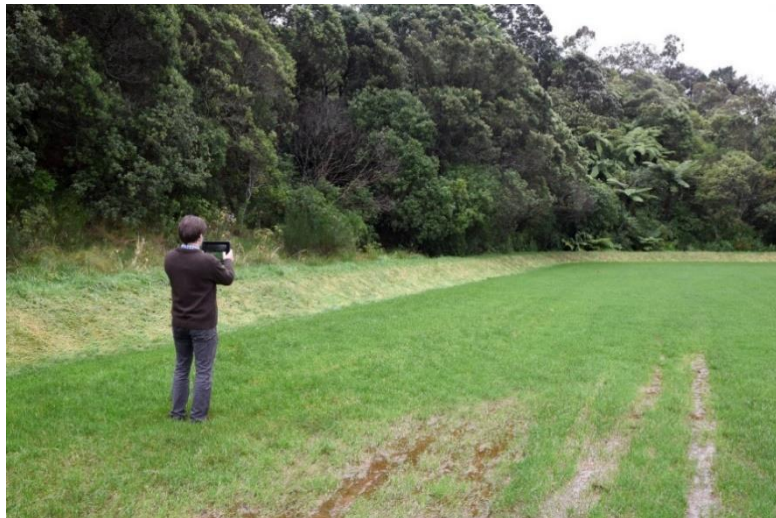
Figure 2 – Papawai Stream Bund showing boggy ground as a result of either over-topping or seepage through the bund wall.
