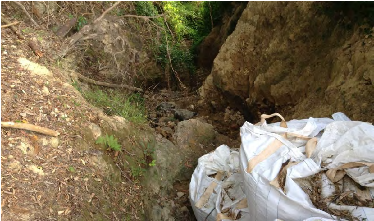
Photo 17: Papawai Stream – Reach 1 showing erosion from flooding.
